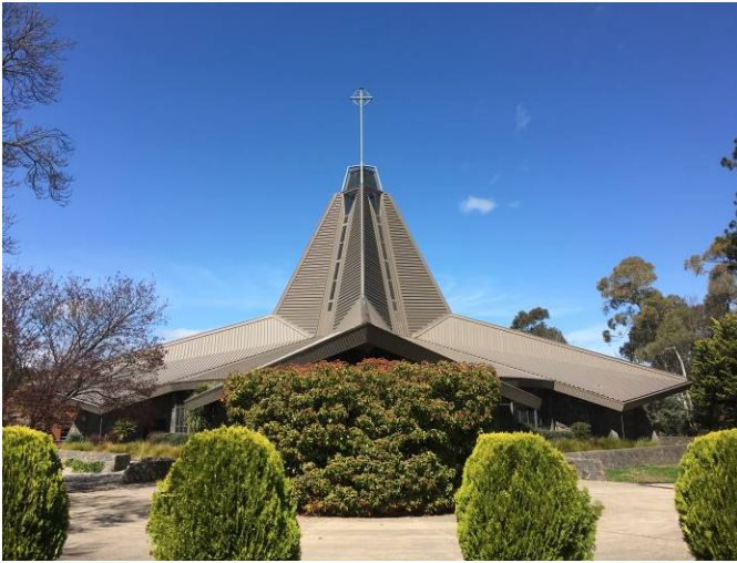
Image 3 Tower, spire and roof folds of St Joseph's Catholic Church (ACT Heritage 2016)
